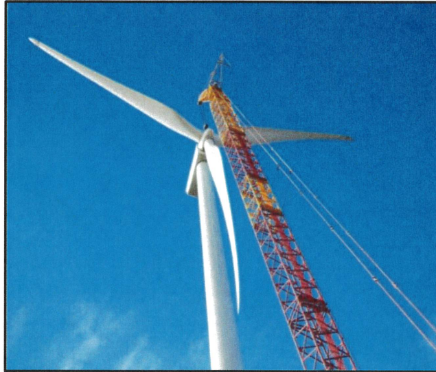
Figure 1.1-1. Example wind turbine.
