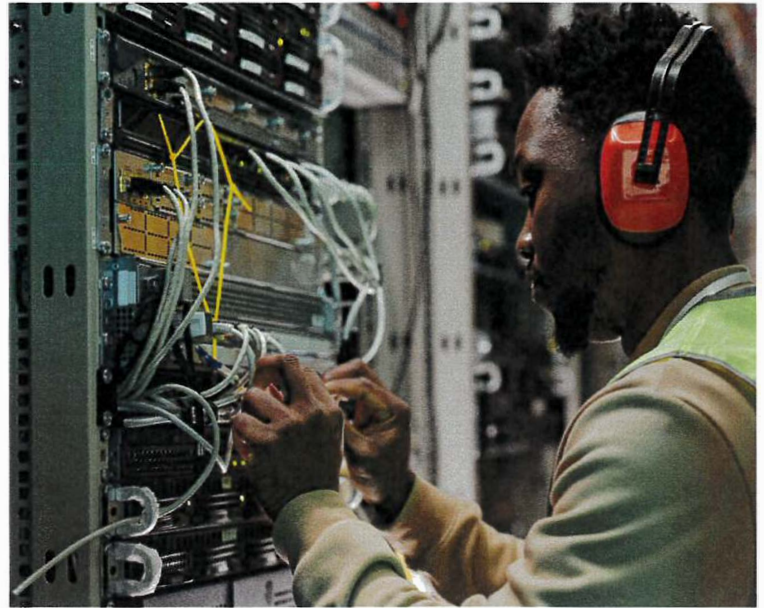
Data centers are filled with servers that emit a consistent and loud white noise.
