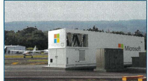
Modular data center. Source: Microsoft.
