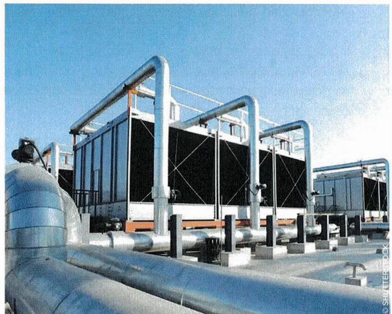
Cooling towers pump large amounts of water through data centers.
