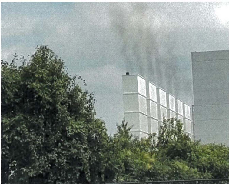
Plumes of diesel smoke arise from a Loudoun fossil-fuel backup generator.
