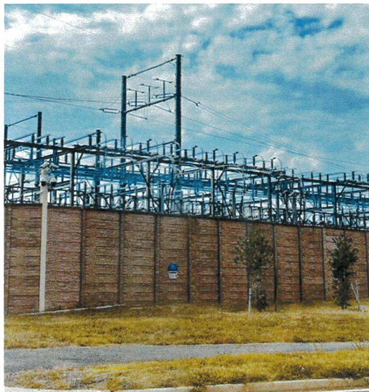
An electrical substation in Ashburn Virginia.
