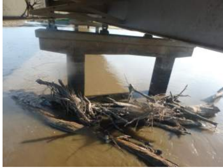
Tree Debris at Bent 2
