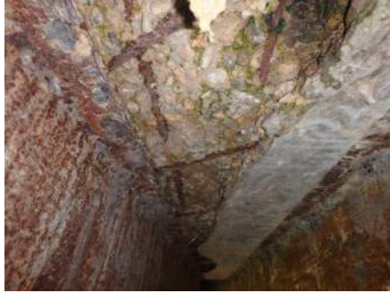
Concrete Deterioration in the Exterior Bays
