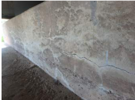
Cracking on Abutment 1 Sill
