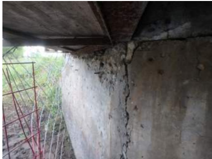
Cracking and Deterioration at the Corners of Abutment 2
