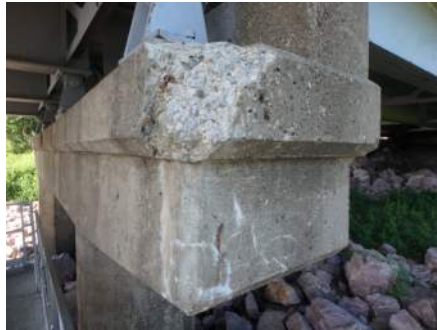
Concrete Deterioration on the North End of Bent Cap 2
