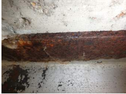
Typical Section Loss on the Top Flange of the Girders
