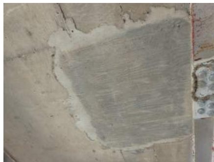
Concrete Patching on the Underside of the Deck at Bolted Splice Locations
