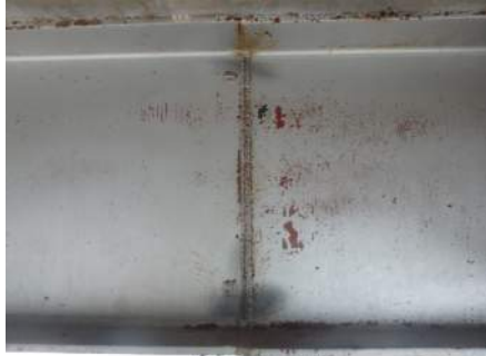
Cracked Splice on Girder 3 in Span 4 West Splice
