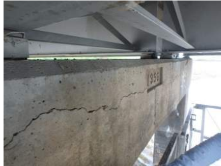
Cracking on the South Face of Bent Cap 6
