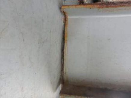
Bulging of Diaphragms from Pack Rust over Bent 5
