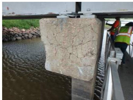
Condition of the West End of Bent Cap 6
