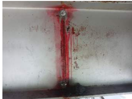
Cracked Splice on Girder 3 in Span 4 West Splice (Testing and Crack Tips)
