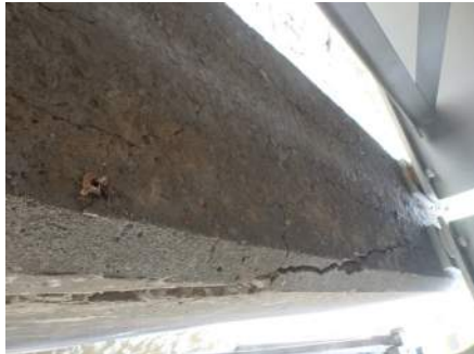
Crack on the Top of Bent Cap 6 East End
