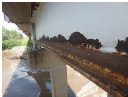
Typical Corrosion to the Exterior Girders
