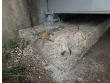
Concrete Deterioration East End of Abutment 1
