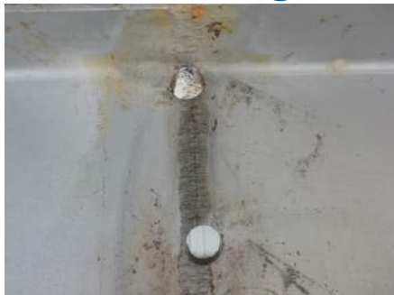
Arrested Crack on Girder 2 Span 3
