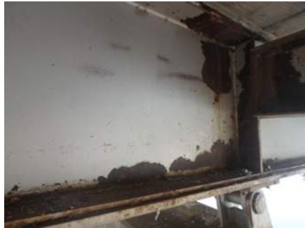
Corrosion of Girders over the Bents
