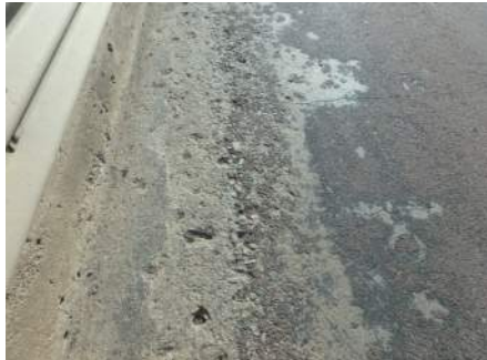
Typical Deterioration of the Edge of the Deck
