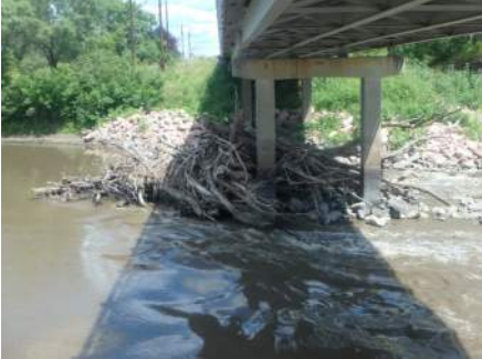
Tree Debris at Bent 5
