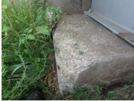
Concrete Deterioration on the West End of Abutment 7 Sill
