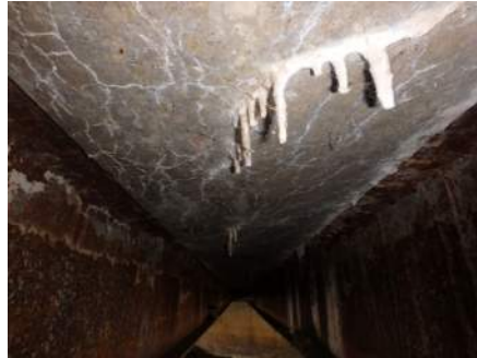
Typical Efflorescence and Stalactites on the Underside of the Deck
