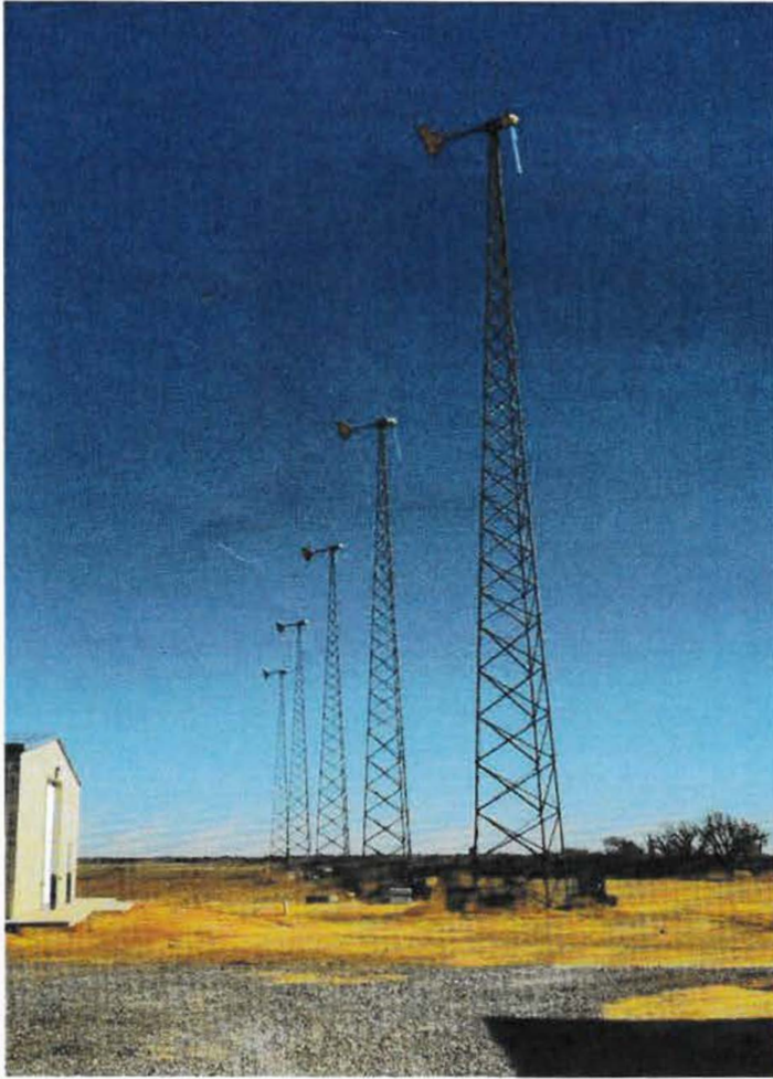
(5) Bergey Excel's on 100' Towers in Drummond, OK
